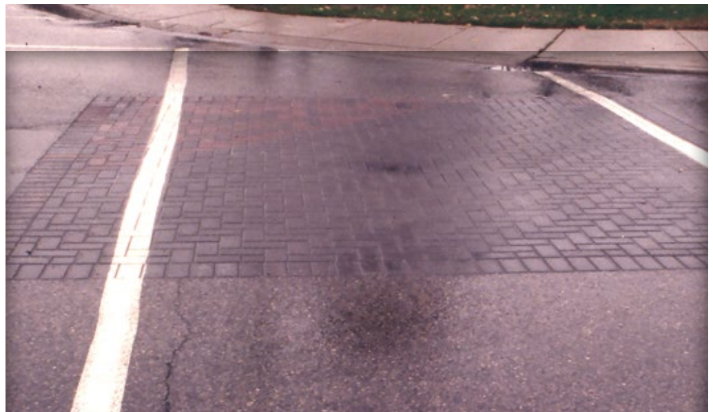
Figure 13. Concrete pavers in utility cuts can be painted as any other pavement.
